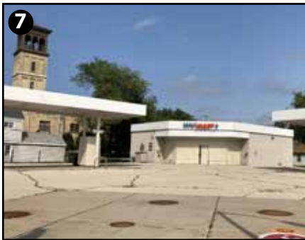
7 171 N Main St Major Improvements Needed
