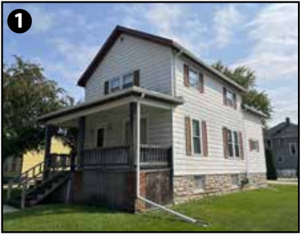
40 W McWilliams St Minor Improvements Needed
