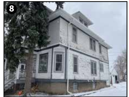
8 22 E Follett St Minor Improvements Needed
