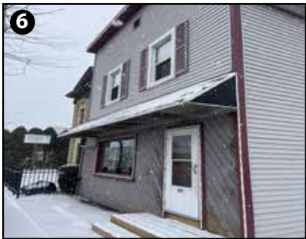
6 191 N Main St Minor Improvements Needed
