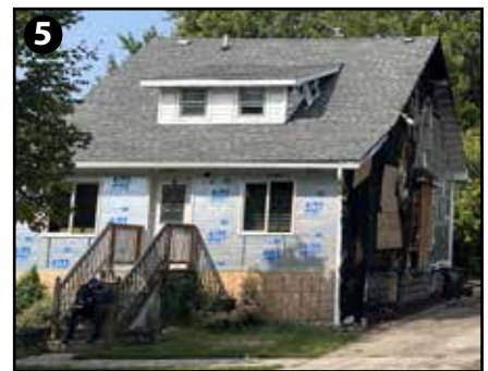
29 W Bank St Major Improvements Needed
