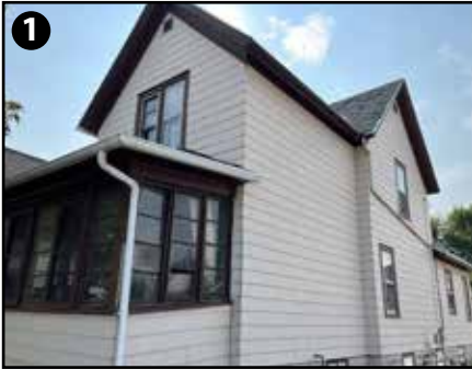
250 N Main St Major Improvements Needed
