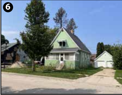
6 15 W Bank St Major Improvements Needed
