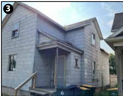
244 N Main St Major Improvements Needed
